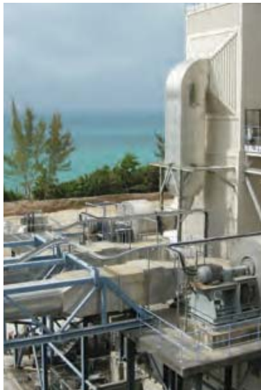
Based on an inspection of Tynes Bay Waste Treatment Facility in Bermuda, Ramboll made proposals for upgrading the facility. We are also consultants for the establishment of a new 72,000 tpa unit.
