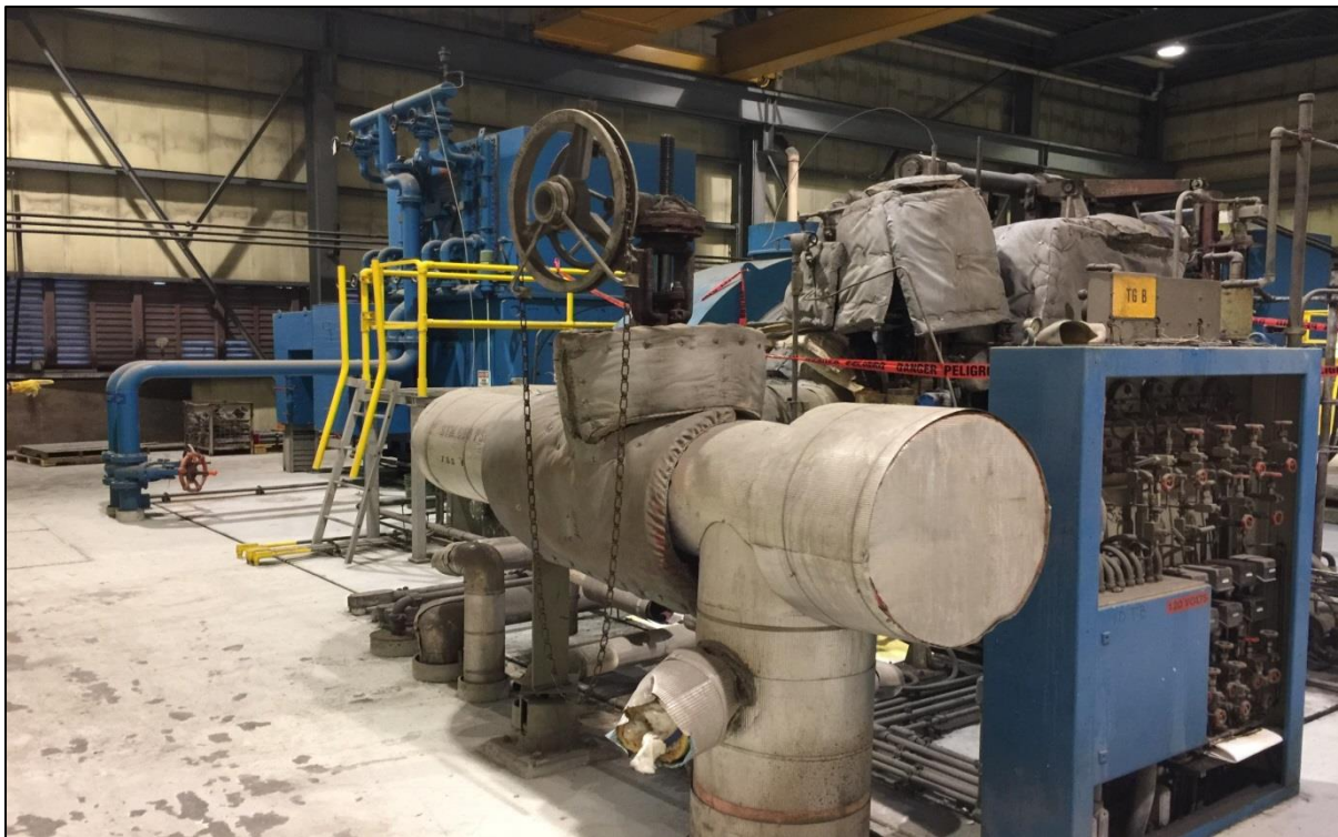
Photograph Covanta Camden Energy Recovery Centre Facility Philadelphia
