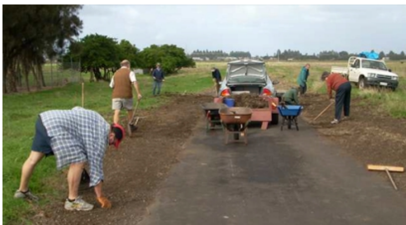
Volunteers organised by the Committee of Management at a busy bee to undertake maintenance work along the rail trail near Port Fairy in Victoria.
