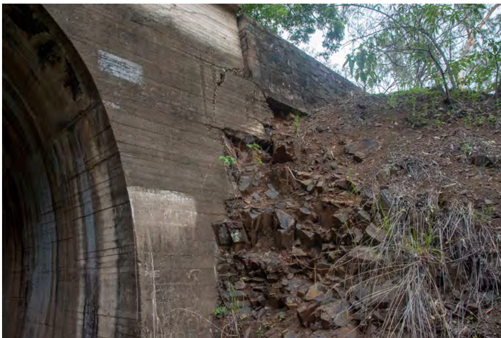
Figure 4. The northern portal of Tunnel 4 has had the wingwall extended using a wall built from stone. This wall, which may have been an informal solution by the builders has moved from earth pressure and broken the concrete to which it was attached.
