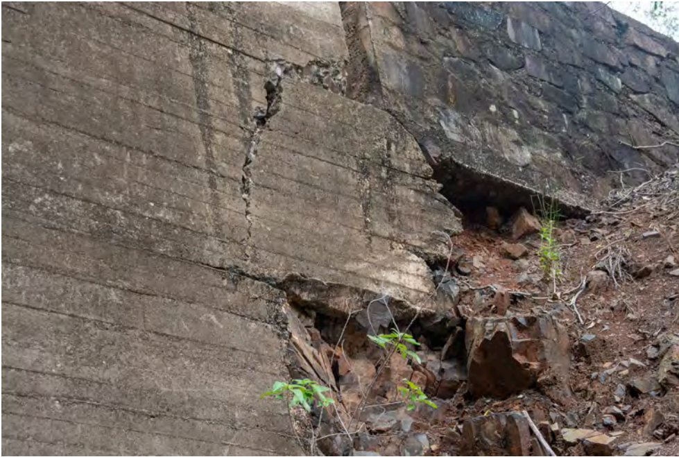
Figure 5. Detail of figure 4. It can be seen that the stone wall on the right has possibly moved outwards and its base undermined. The movement has taken part of the concrete headwall with it.
