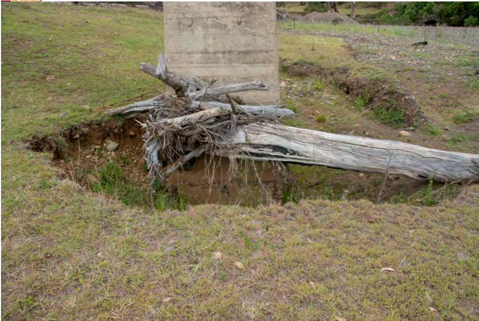
Figure 9: Scour around pier base at Glassford Creek. If the pier is founded soundly on rock, risk is low. Otherwise rip-rap could be dumped to limit further scour.
