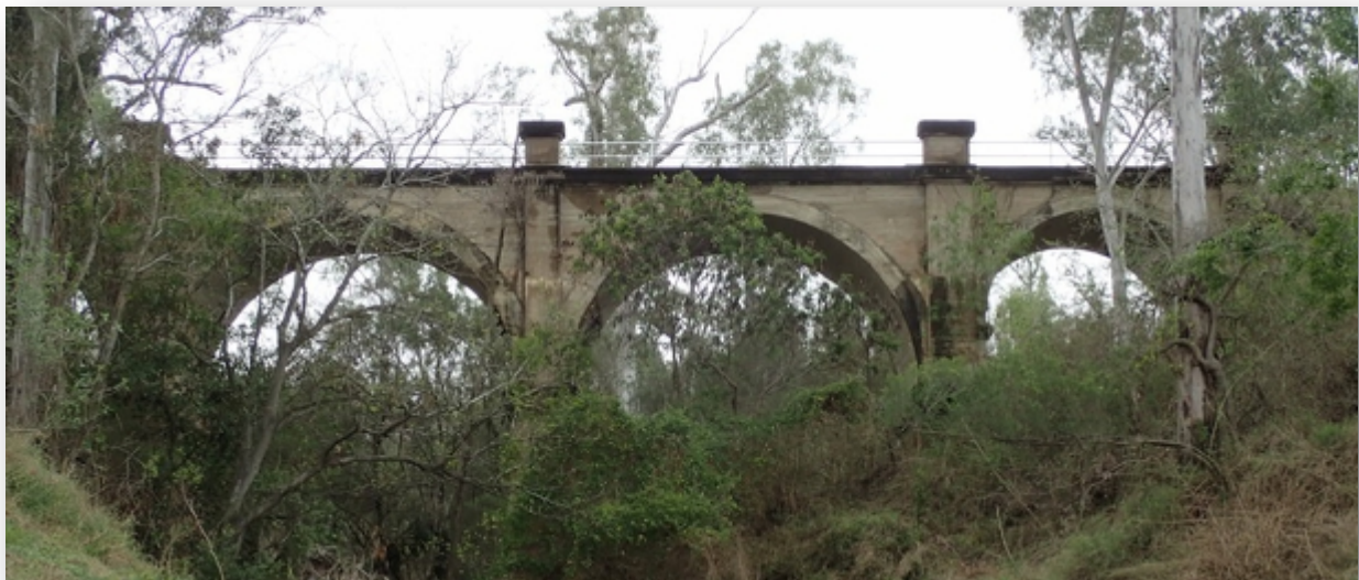
The historic and heritage listed bridges between Mundubbera and Gayndah are a major factor influencing the attractiveness of this section of disused railway corridor for development of a standalone rail trail.
