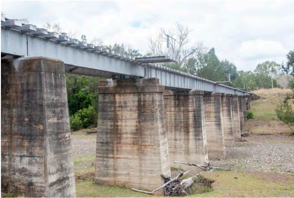
Figure 7: Glassford Creek bridge. The superstructure of the centre seven spans are made from rivetted plate web girders; three spans on each end use compound girders with flange plates rivetted top and bottom. Changes in the pier tops also suggest that the bridge was lengthened after the original construction.
