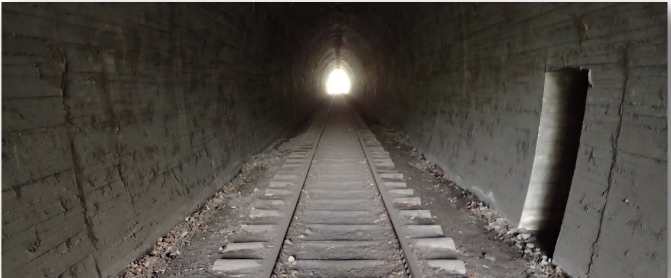
Retention of the unique hog's back timber railway sleepers within the tunnels is one of the key factors to be considered when developing the rail trail.
