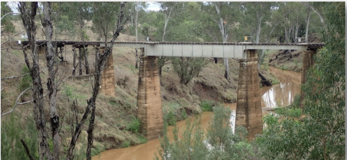
Many of the bridges traverse steep and deep creek valleys. Retention of the bridges is far preferable to construction of a lower level crossing.
