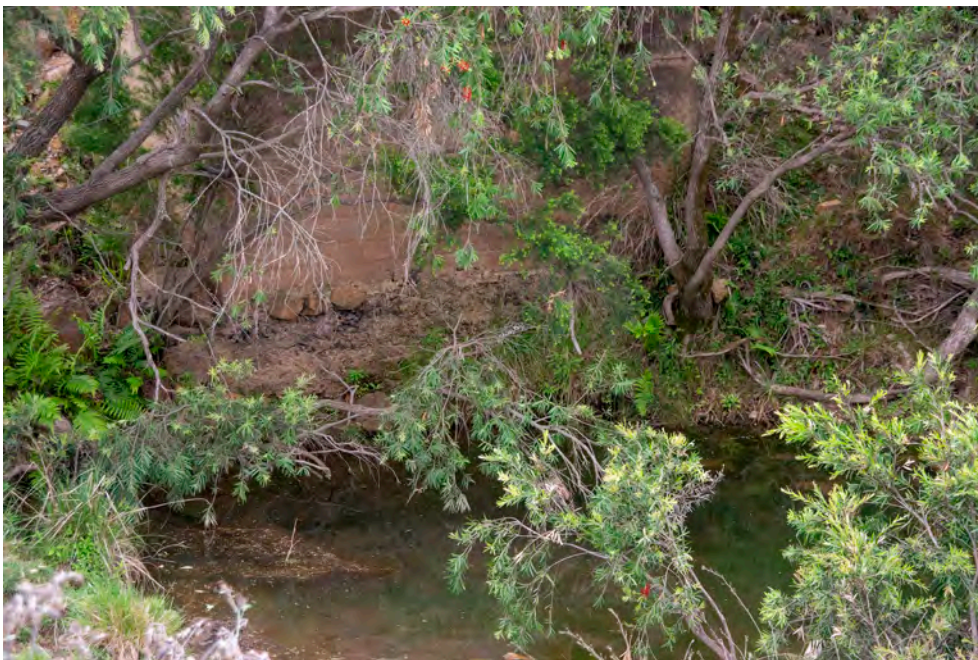
Figure 8: Pier base in small creek at underbridge. The founding of this pier needs to be checked against drawings and rip-rap may be needed to limit future risk from scour.
