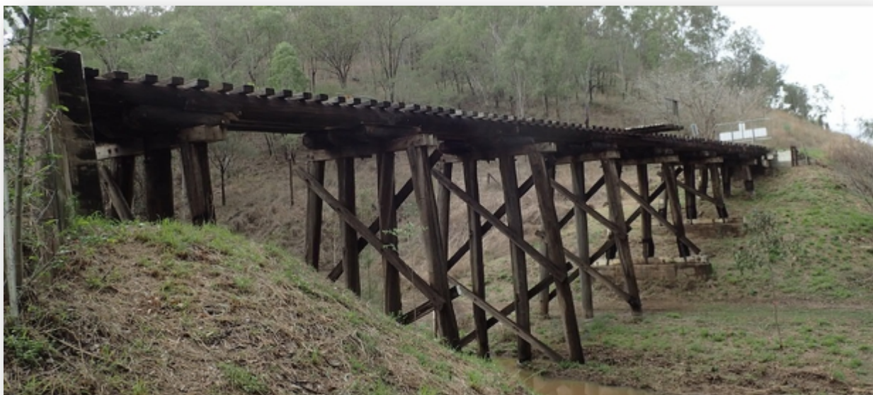
Many of the timber bridges have been removed from the corridor: however, some of the most strategically positioned bridges have been retained for future rail trail use.
