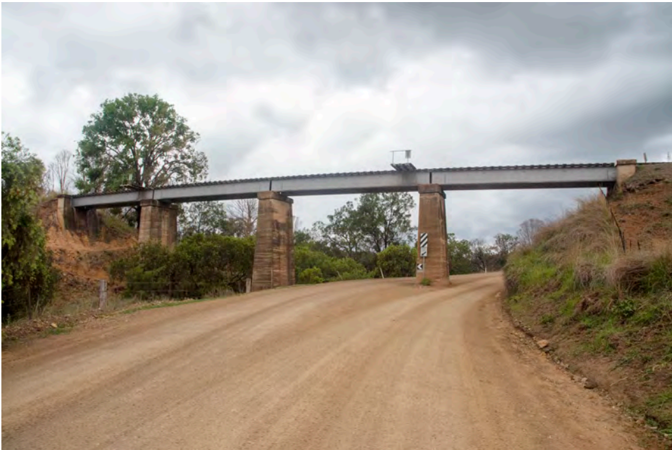
Figure 6: Underbridge north of Kalpowar. The bridge uses welded plate web girders, which may be a modern replacement for an older superstructure as such girders were not used at the time of the original construction
