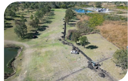
$2.2M Calliope Wastewater Treatment Plant irrigation
