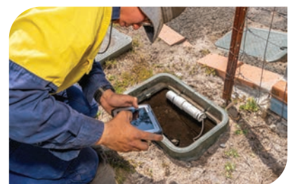
$1.1M Advanced metering infrastructure at Lake Awoonga
