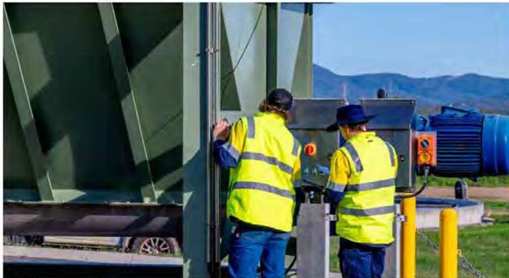
Gladstone waste water planned maintenance
