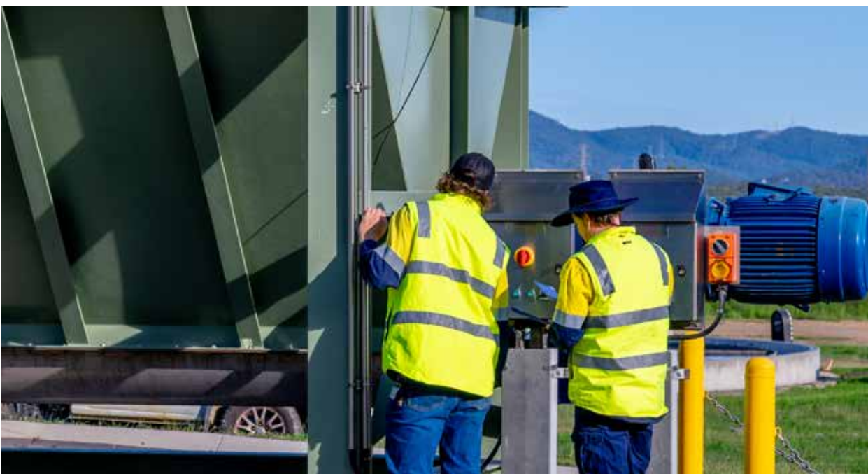
Gladstone waste water planned maintenance
