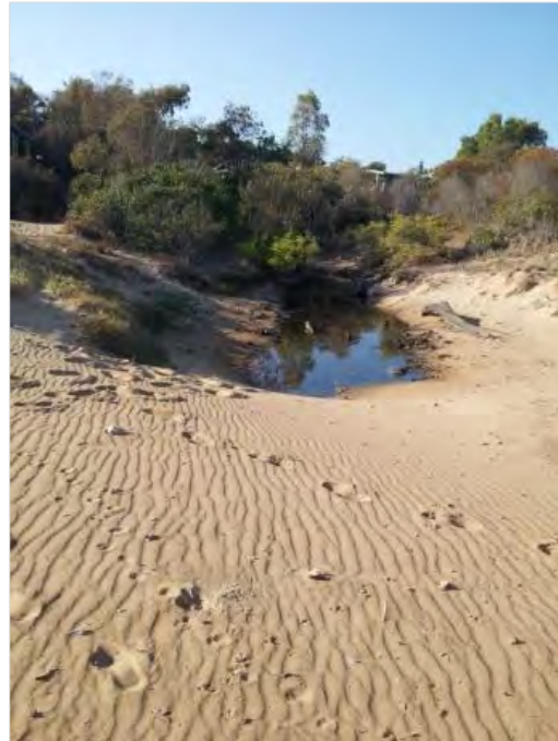
Plate 10 - Stormwater drainage blocked by deposited sediments
