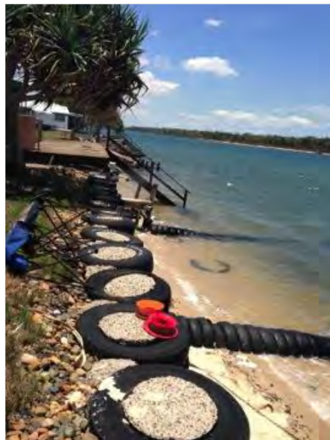
Plate 16 - Erosion structures made of various materials and designs installed by residents on the mainland side of Colosseum Inlet
