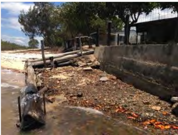
Plate 15 - Revetment walls installed by residents on the mainland side of Colosseum Inlet
