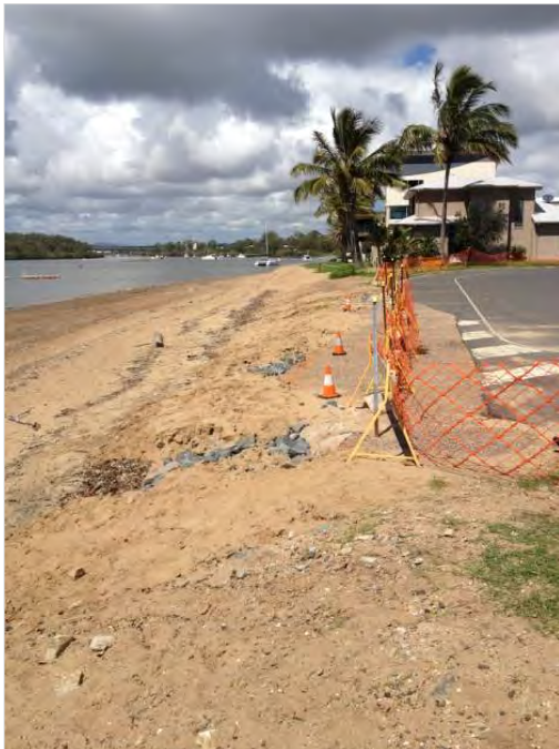
Plate 8 - Barricade along edge of scoured car park showing sand replenishment
