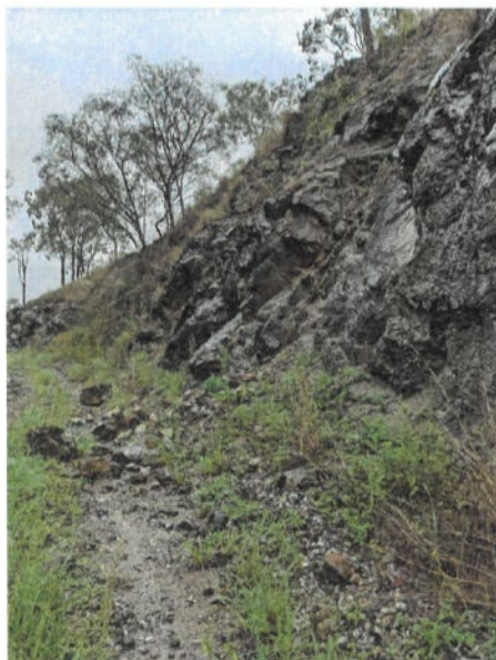
Typical rock cutting with rockfall evident
