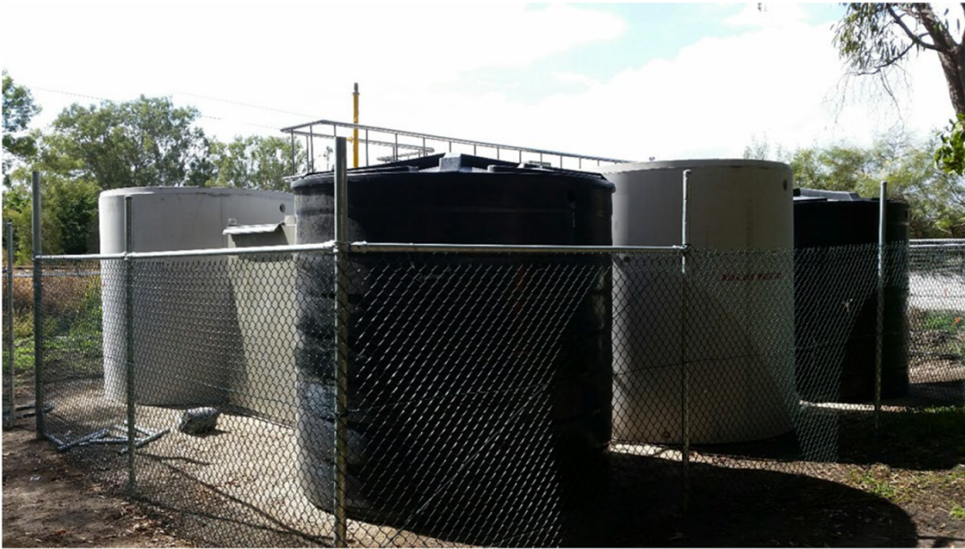
Figure 1 – Alf Larson Wastewater Treatment Plant
