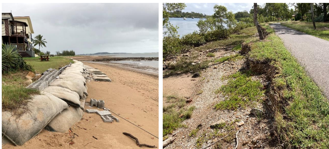
Figure 7-1: Field investigation of erosion at Island Esplanade (left) and Turtle Way cycle path (right)
